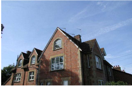
82. Unsightly clutter of aerials facing the highway
